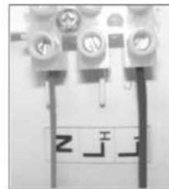
Wiring Photograph: Low Speed
